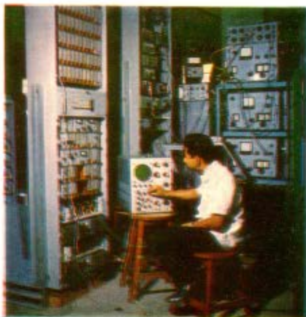
Coaxial Transmission Equipment under test
