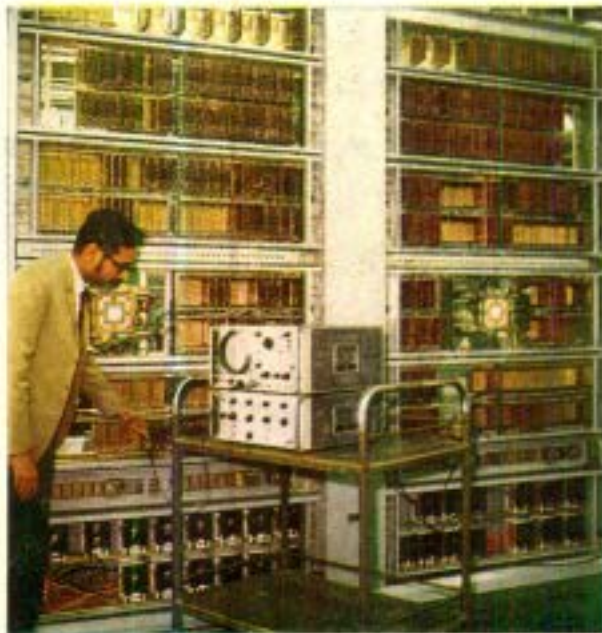
Electronic Exchange Equipment on test
